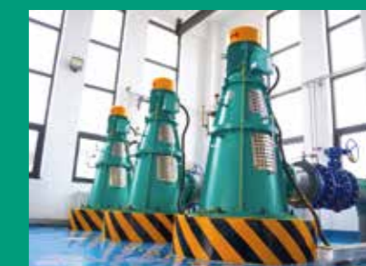
Wilo technology is in operation at a waterworks in Xiong'an.
