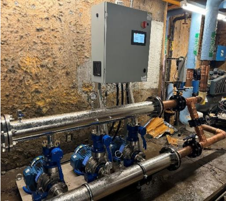
Newly installed Wilo-WiBooster at Austin, Texas hotel
