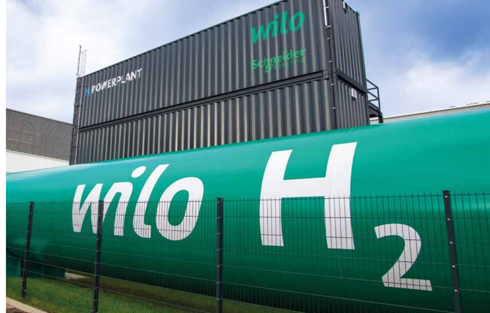
The H 2 POWERPLANT pilot hydrogen facility at the Wilopark, the company's headquarters in Dortmund, is an important element of the Wilopark energy concept, as it stores the electricity generated by the photovoltaic system on the factory roof and then distributes it when it is needed.
