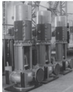
Vertical Sewage Pumps
