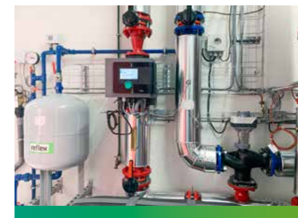
Using heat from compressed air generation at the production site in Laval, France
