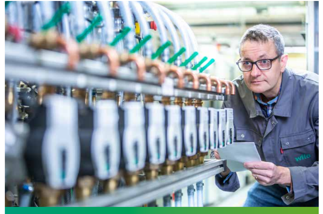
Service life test of highly efficient OEM-pumps in Aubigny, France
