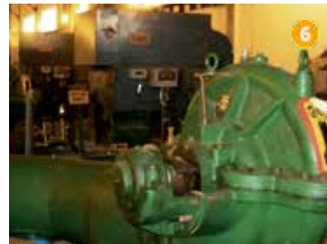
Supply of drinking, process and cooling water, blow down pumps and settling tanks, SSF Feed pumps Steel Ltd., Jam- shedpur, Jharkhand, India
