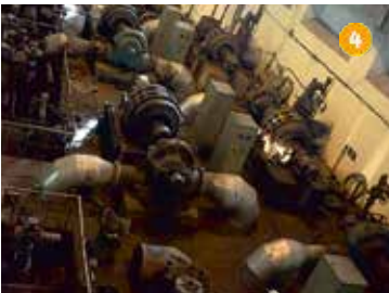
Water transport and cooling water, Steel Plant Bhilai, Chattisgarh, India
