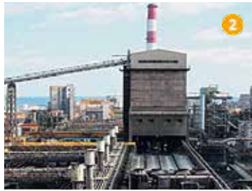
Water jet door cleaning system in cokes utility, raw water intake, water transport, Steel Manufacturing, Pohang, South Korea
