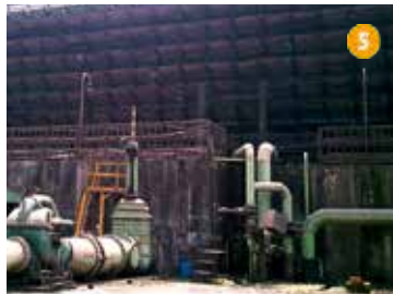
Cooling towers, ispart, steel producer/ hot rolled coils, Dolvi, Alibaug, Maha- rashtra, India
